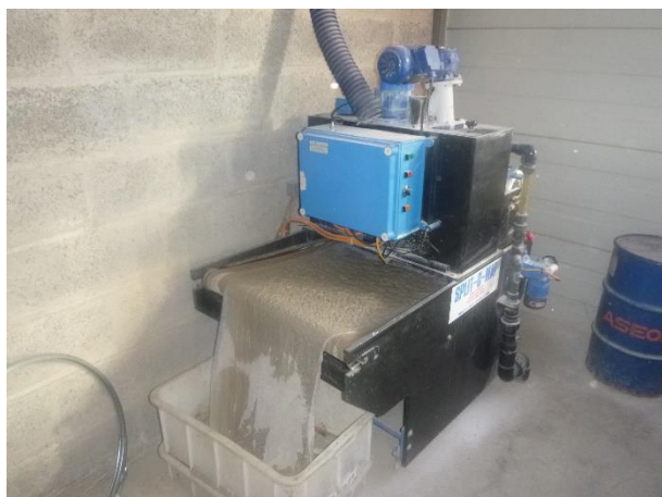
Installation de floculation
